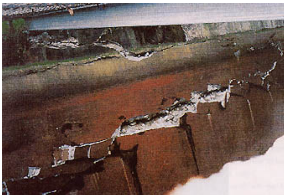
Photo 5 Damage to open aqueduct
