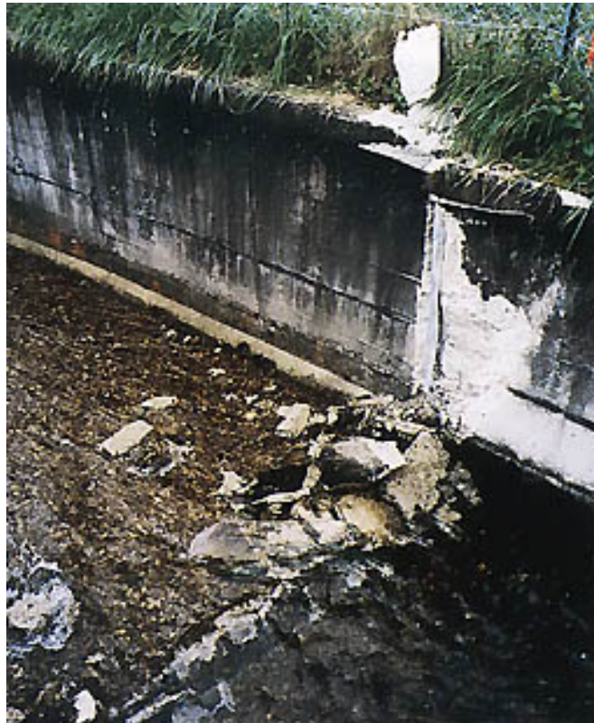
Photo 2 Damaged concrete wall of drain
