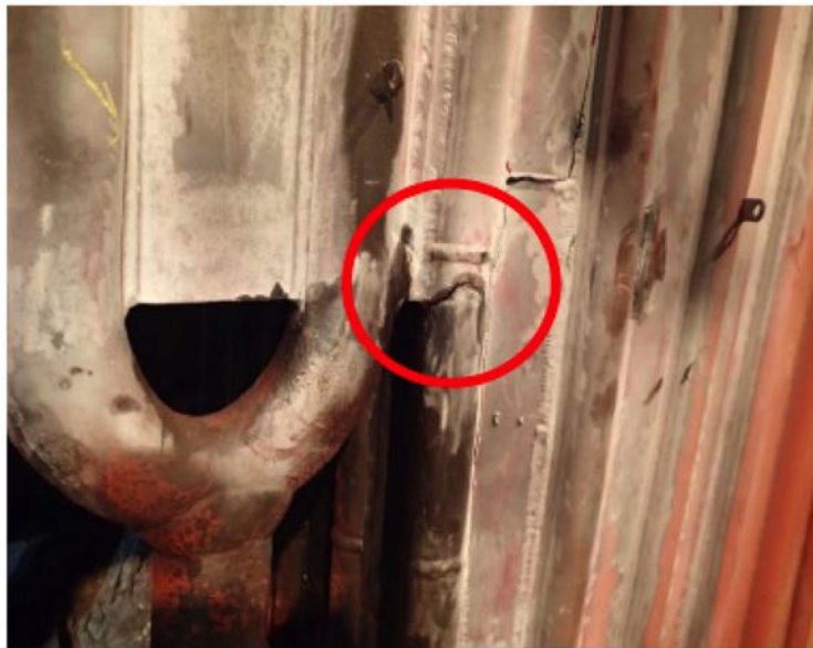
Unit 1: Boiler tube damage situation
