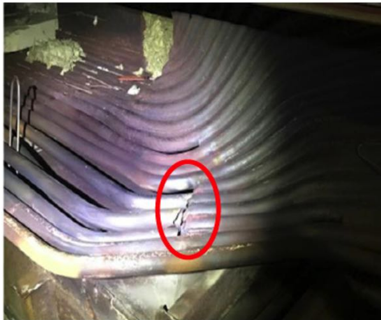
Unit 2: Boiler tube damage situation. ①
