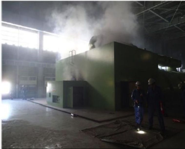
Unit 4: Turbine fire condition
