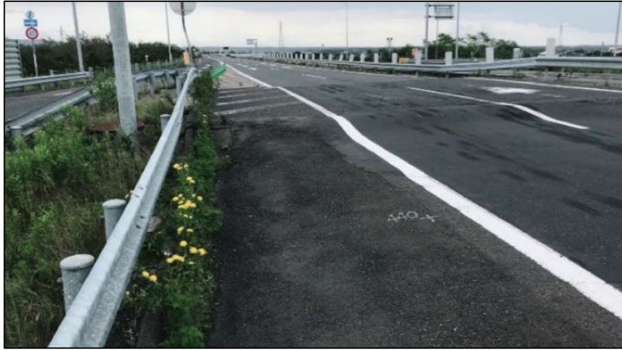
Figure 7-21. Mukawa Interchange area road surface damage. (Credit: MLIT)
