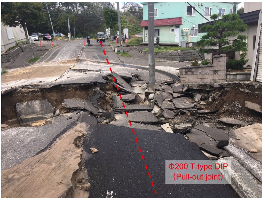
Figure 5-9. Damage to 500 mm DIP Pipe (credit: Kubota)
