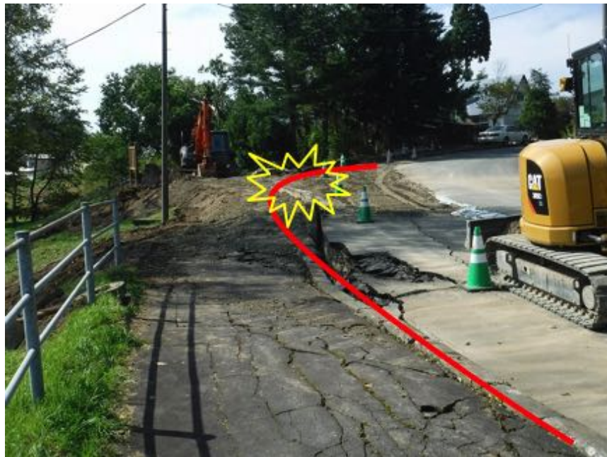
Figure 5-18. Location of damaged 150 mm PVC Pipe (credit: Kubota)
