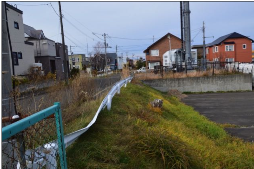
Figure 6-14. Guard Rail twisted and support poles rotated
