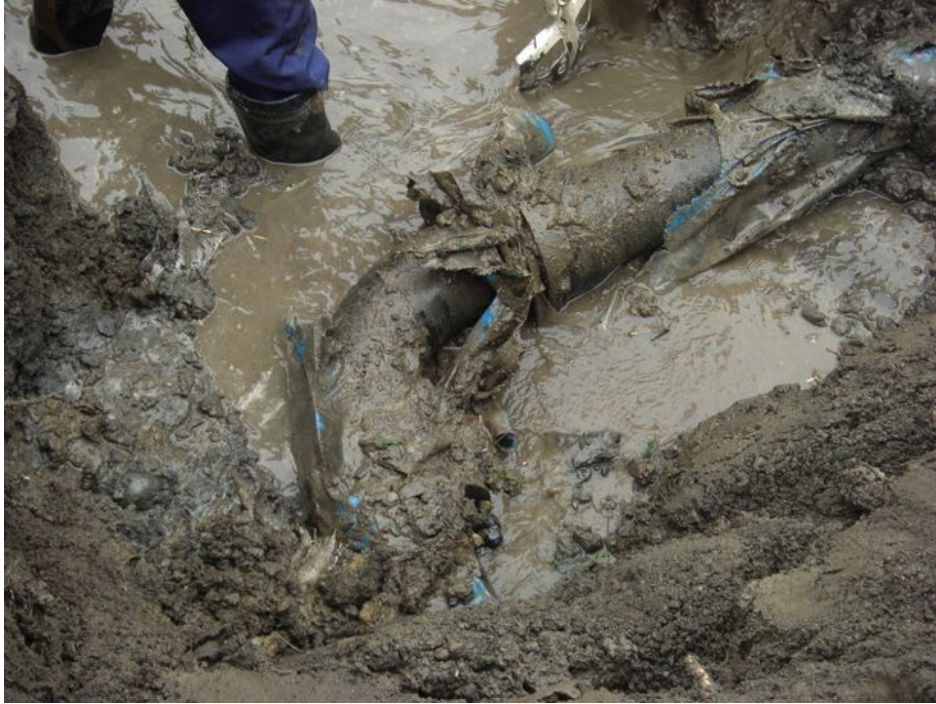
Figure 5-21. Pull-out of K-type joint for 150 mm DIP near road embankment slip in Figure 5-17 (credit: Kubota)
