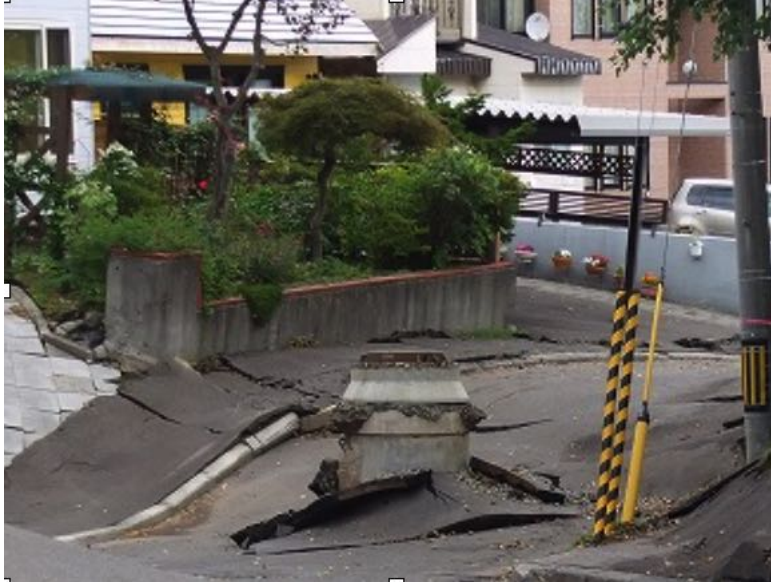
Figure 5-10. Manhole in Liquefaction Zone (credit: Kubota)
