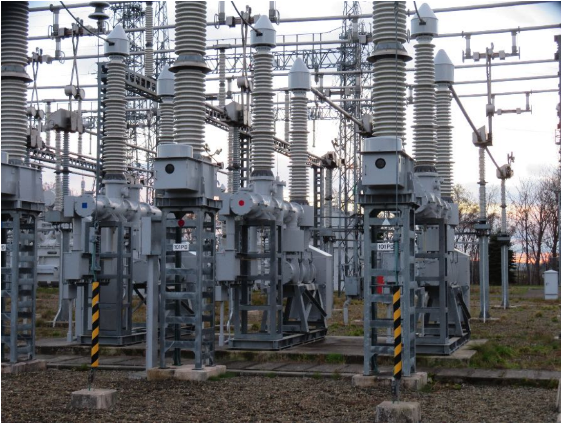
Figure 3-10. Eniwa 187 kV Substation. 187 kV Circuit Breakers
