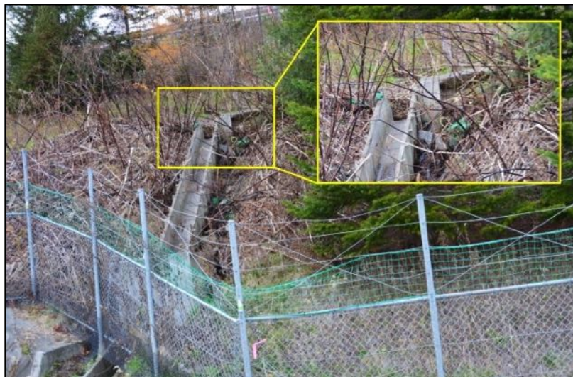
Figure 6-5. Evidence of ground deformation at the abutment area, ~ 30 cm displacement of the drainage channel.
