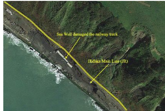
Figure 7-6. Wave damaged the sea wall, then the sea wall damaged the track. (Google Earth)
