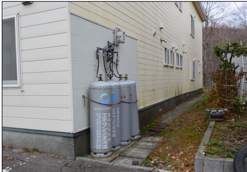
Figure 4-9. Propane tanks strapped to wall anchors. This household uses both gas and propane
