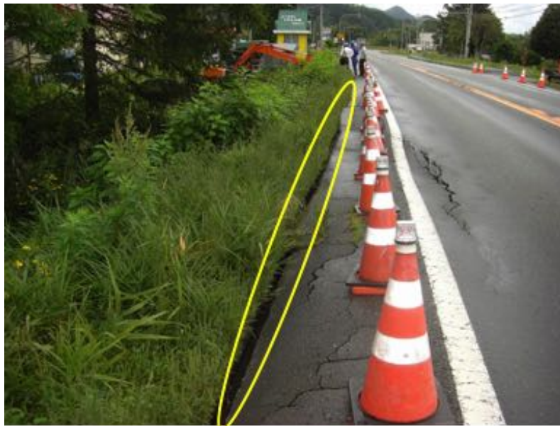
Figure 5-20. Slump of roadside embankment in Biratori-town (separation at edge of asphalt is about 5 inches) (credit: Kubota)
