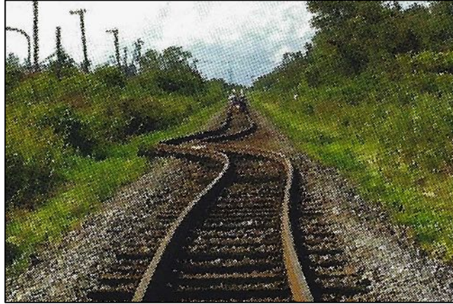
Figure 9-2. Buckled JR track on Hidaka Line. (Source: JR)
