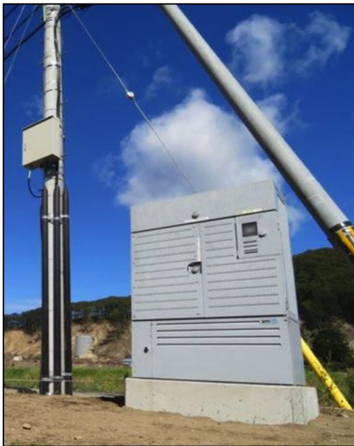
Figure 6-8. The new DLC cabinet, note the water tank of the WTP after the landslide (Source: Prof Suzuki of Toyo University)
