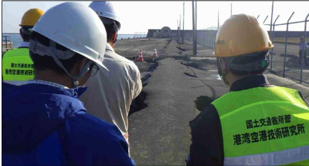
Figure 8-12. Tomakomai Port pier liquefaction damage. (Credit: Hokkaido MLIT)
