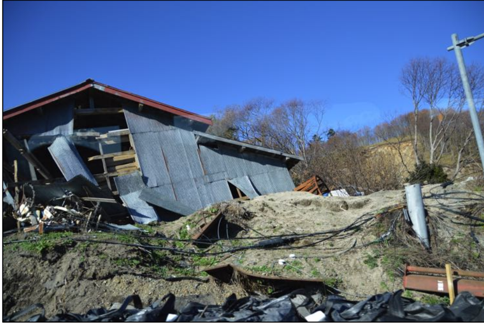
Figure 6-2. Telecom poles and cables (metal and fiber) destroyed by debris
