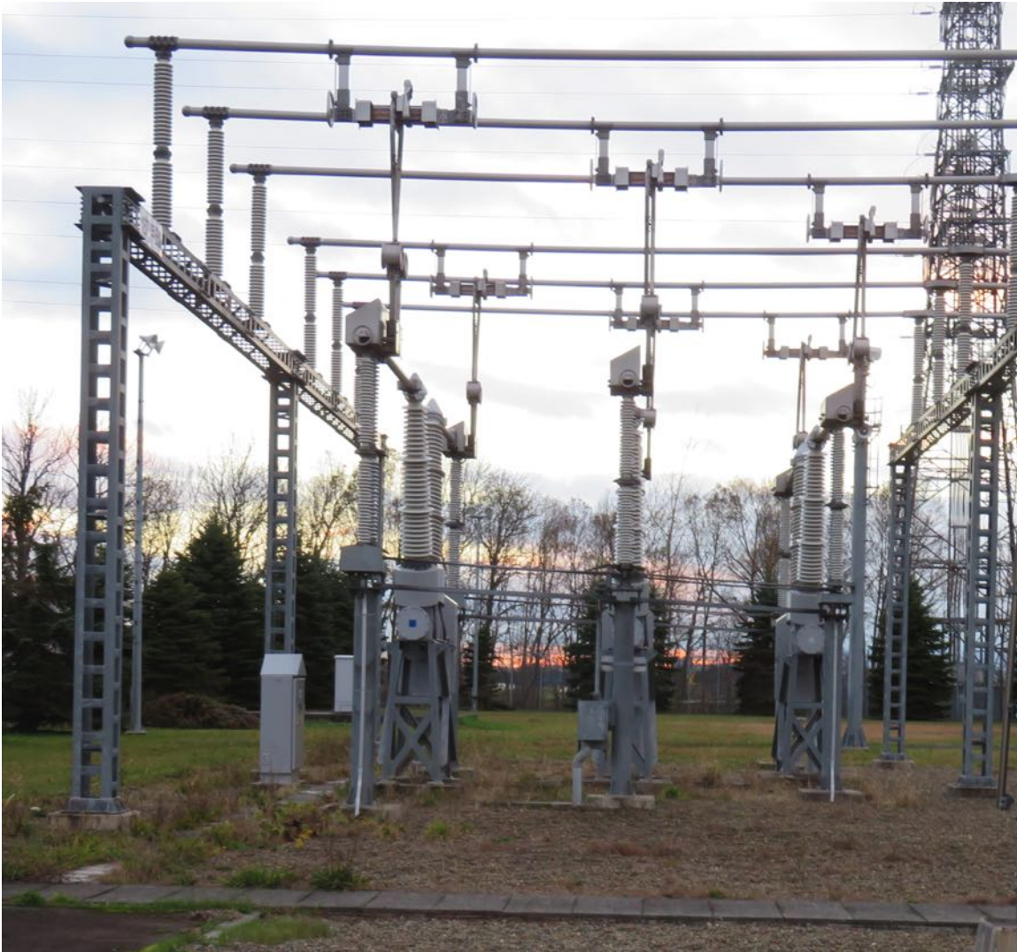
Figure 3-11. Eniwa 187 kV Substation. 187 kV Pantograph Switches
