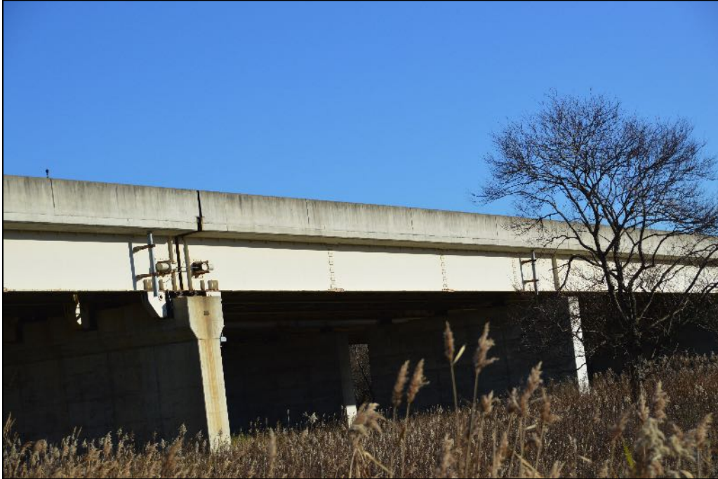
Figure 7-25. The deck slide prevention key and the cable tying the decks provided a suitable measure to avoid unseating of the road decks at this location
