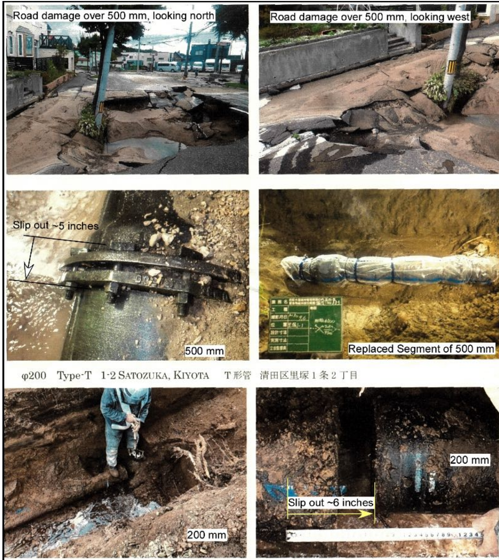
Figure 5-7. Pipe Damage in the Liquefaction Zone (credit: City of Sapporo)
