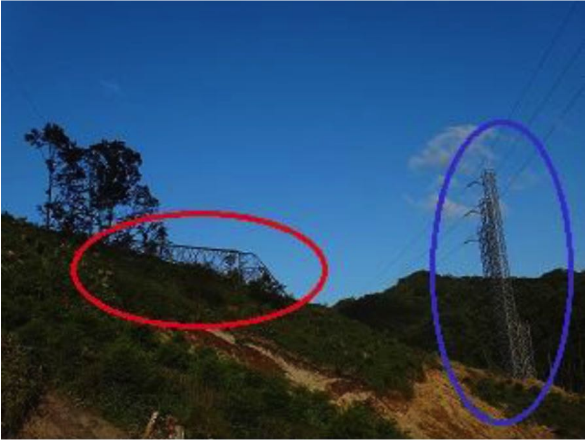
Figure 3-29. Collapsed Tower 107 (Red Circle) and Replacement Tower (Blue Circle) (photo: HEPCO)
