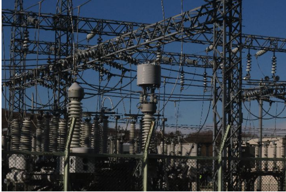
Figure 3-15. Hayakita 66 kV SF6 Wave Trap
