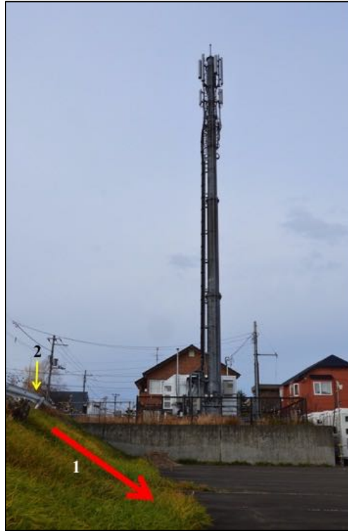
Figure 6-13. This site shows a slight slide (1) of surface soil covering part of the parking lot. The guard rail pole (2) was rotated.
