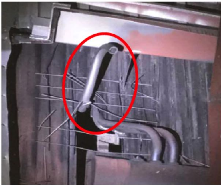
Unit 2: Boiler tube damage situation ②
