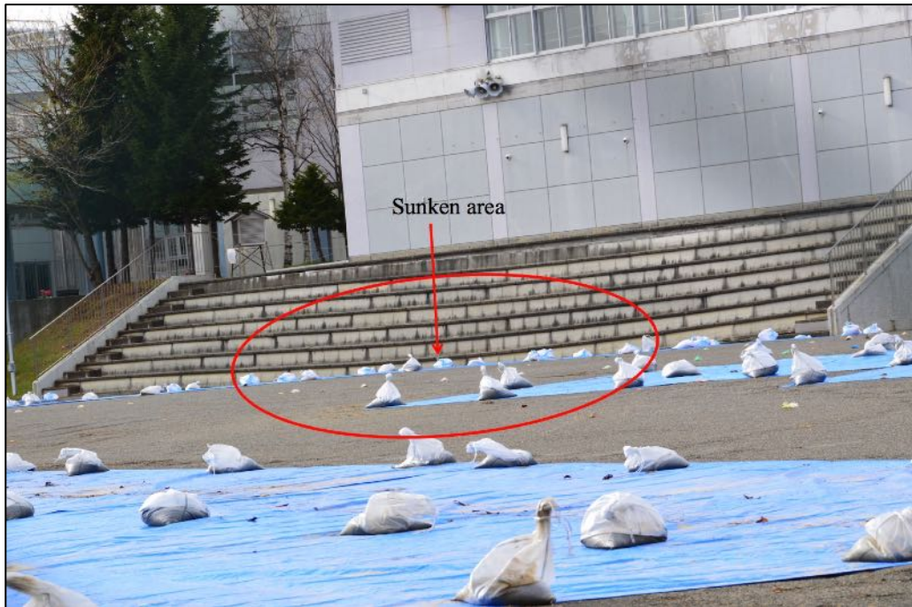
Figure 9-7. Outdoor sports field damaged due to permanent ground deformation
