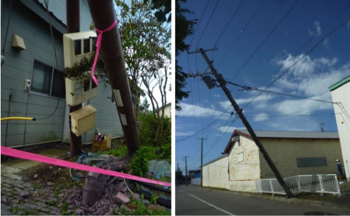
Figure 3-46. Toppled and Tilted Distribution Poles (Credit: HEPCO)
