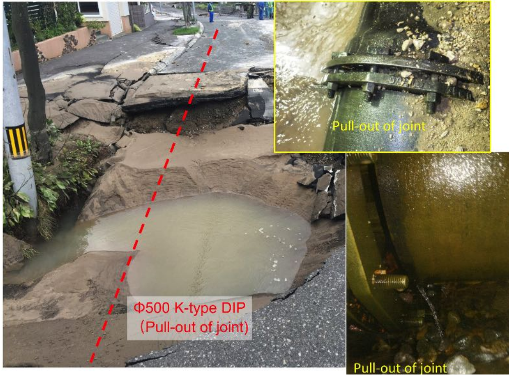
Figure 5-8. Damage to 500 mm DIP Pipe (credit: Kubota)
