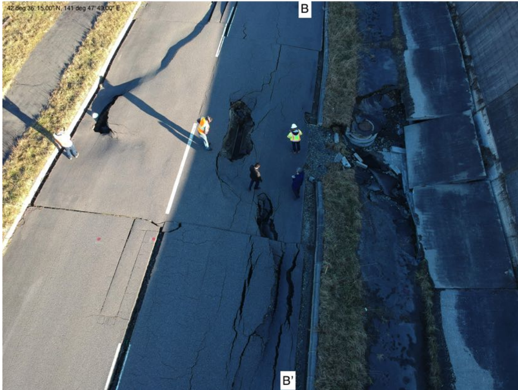
Figure 2-22. Road Failure, Line B-B'
