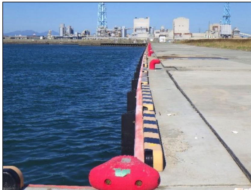
Figure 8-11. Bulging of the quay wall at Tomakomai-Atsuma Power Plant
