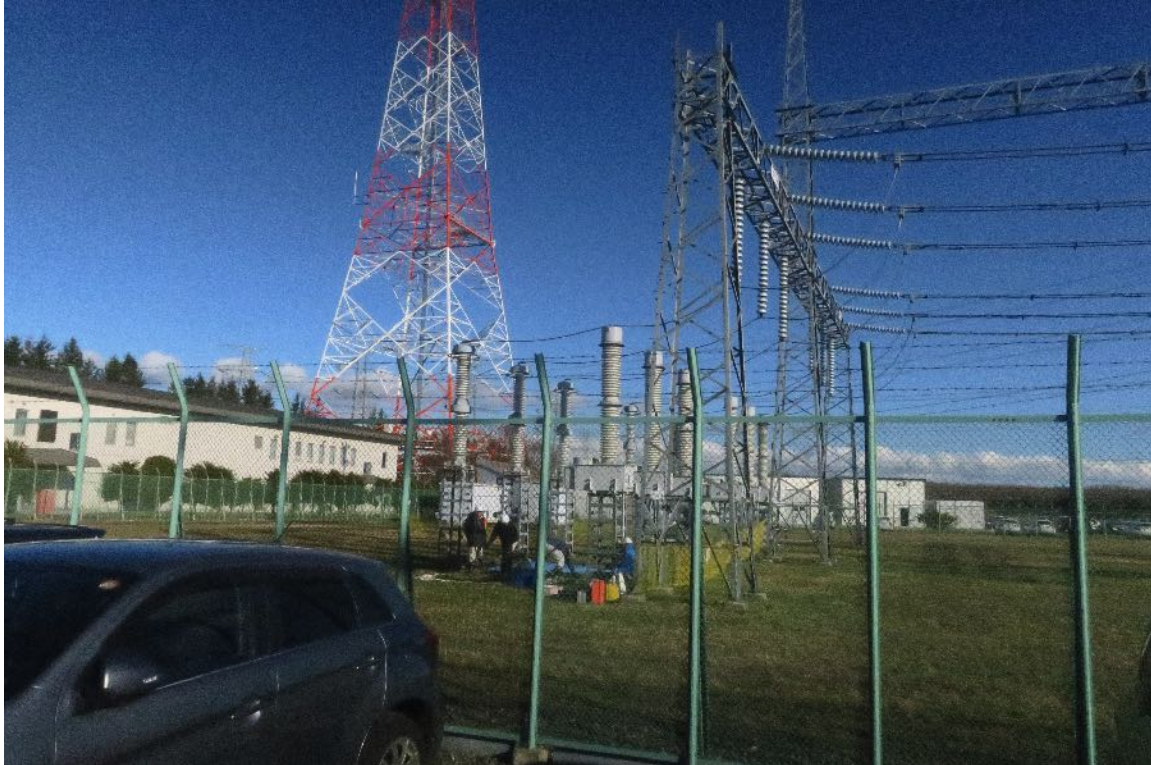
Figure 3-8. Minami 187 kV CCVTs
