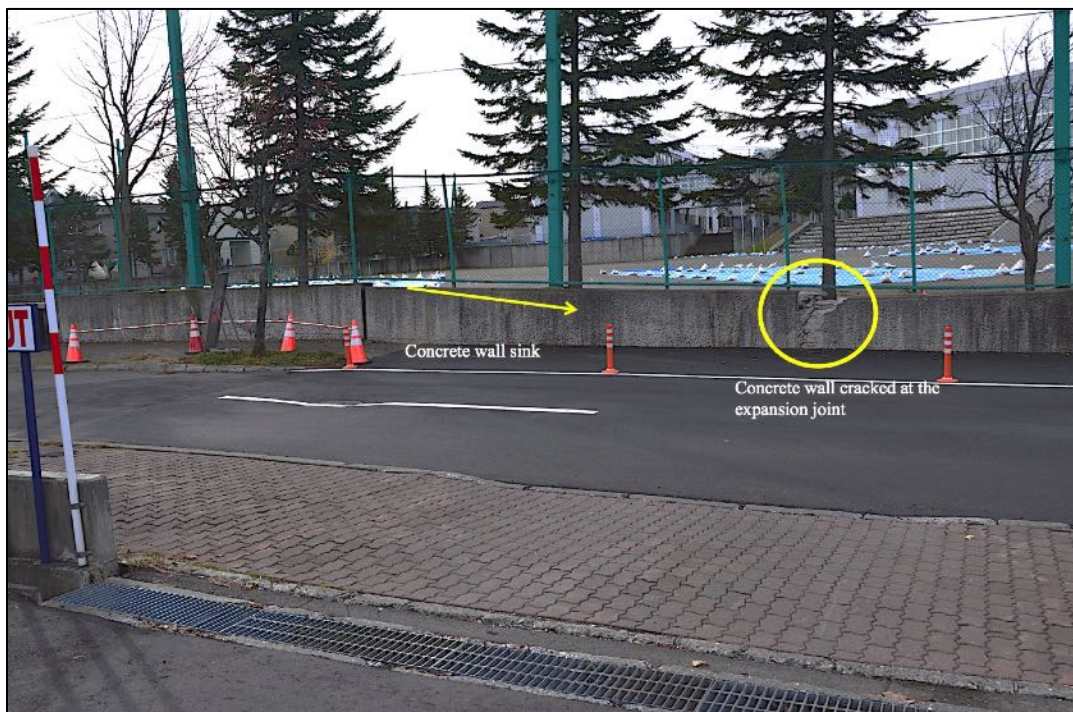
Figure 9-8. Concrete wall broken due to permanent ground deformation
