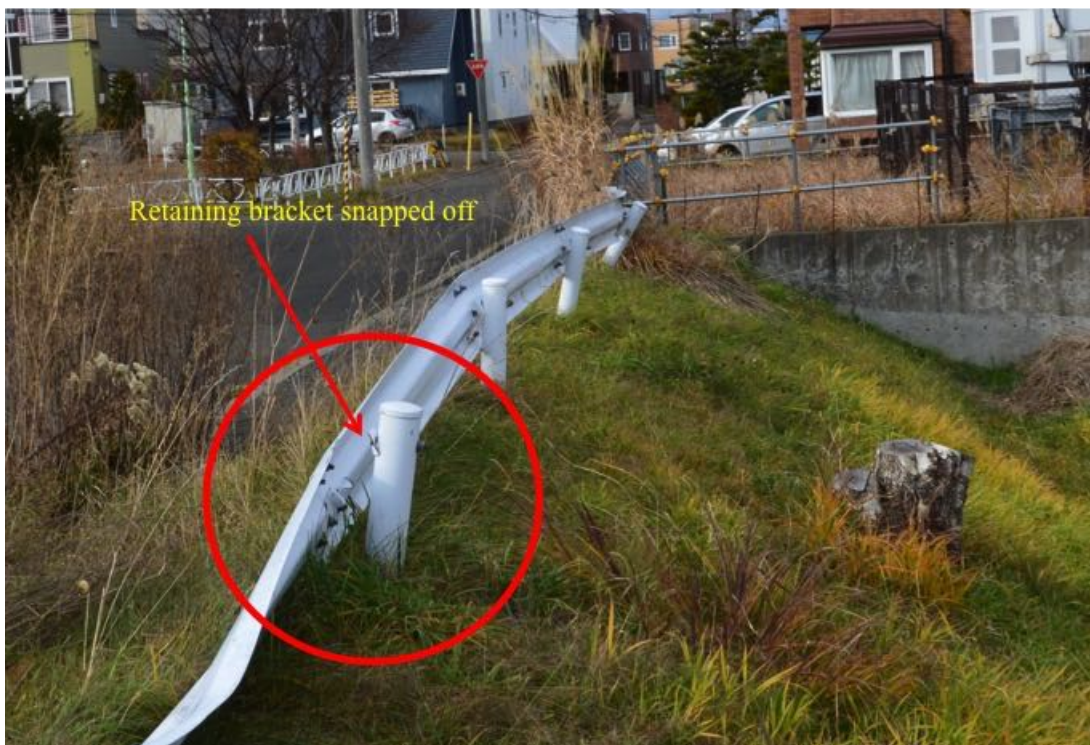
Figure 6-16. Retaining bracket broken from the anchor on the pole.
