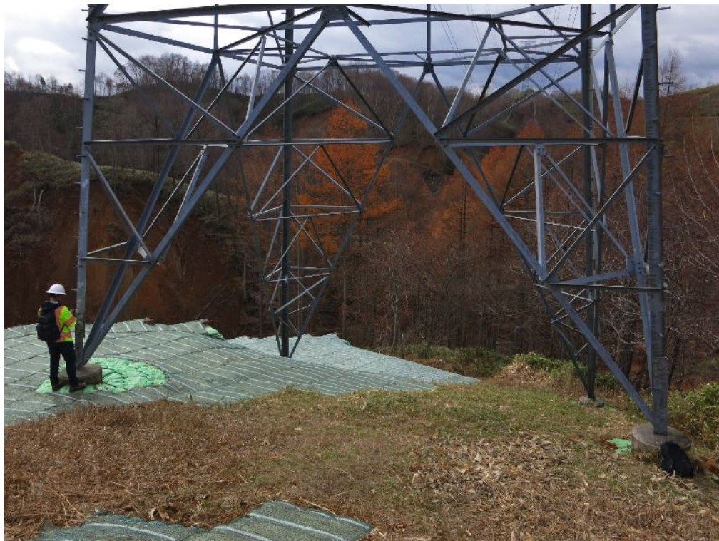
Figure 3-24. Legs and Foundation of Tower
