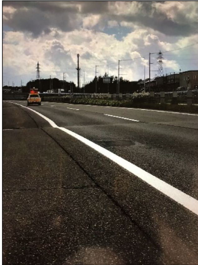
Figure 7-18. Road surface crack close to toll booth at Kita-Hiroshima Interchange. (Credit: Prof Maruyama)
