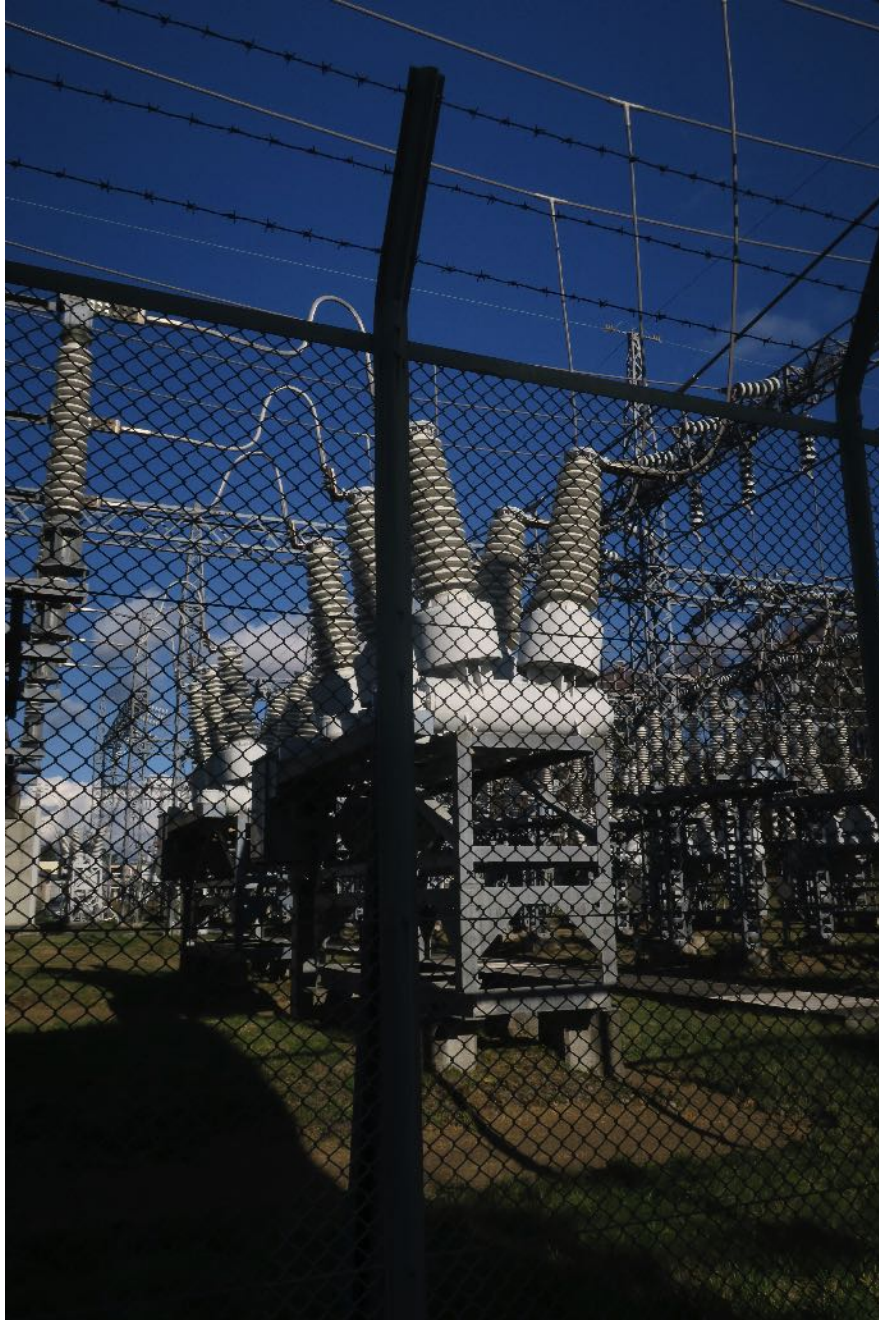
Figure 3-14. Hayakita 66 kV SF6 Circuit Breaker
